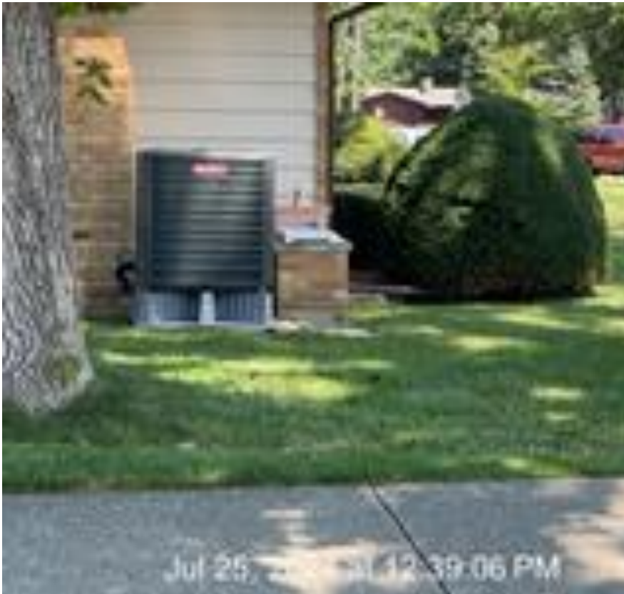
New equipment installed without permit - found in July 2024. Equipment appears to be larger than previous equipment on property.
