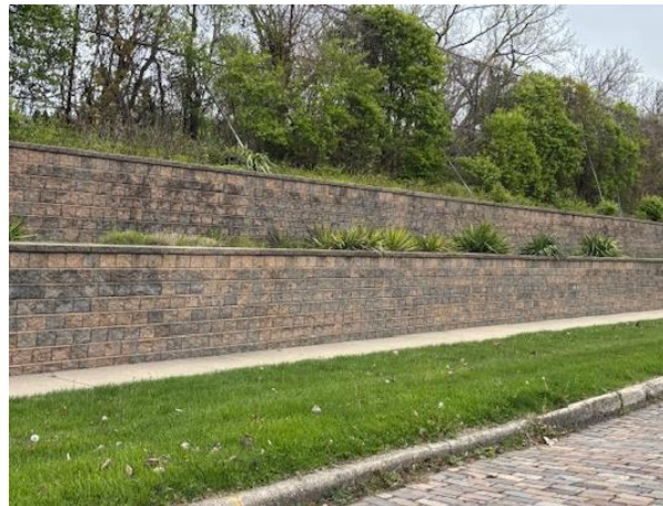
Landscape block two-tiered retaining wall
