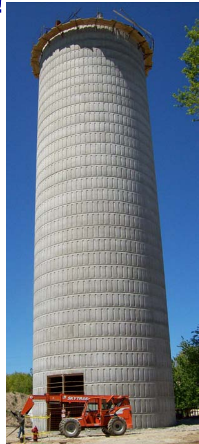
Above: Pedestal for new Authority Water Tower located in Lincoln Charter Township off Jericho Road. Photo courtesy of Wightman and Associates.
